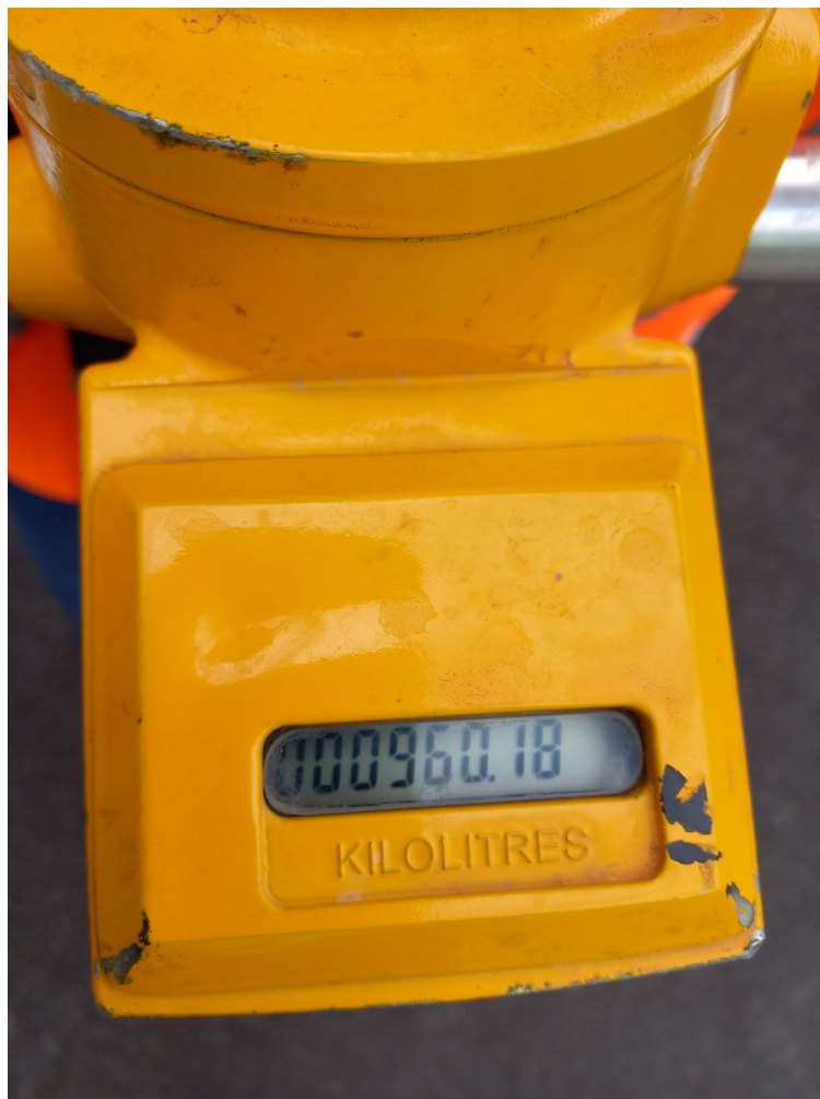
Example Photograph of a Standpipe's Digital Meter
