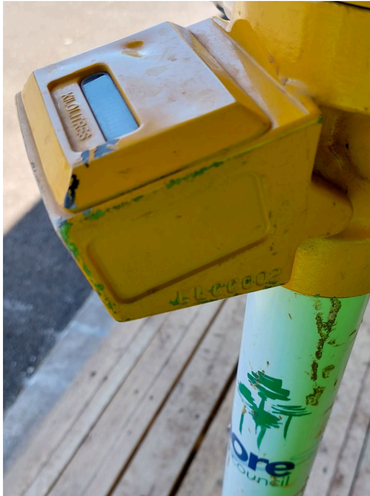
Example Photograph of a Standpipe's Serial Number (Above reads LLCC002)
