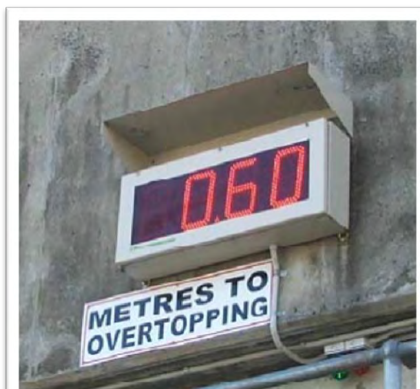
BROWNS CREEK PUMP STATION AT LEVEE SPILLWAY
