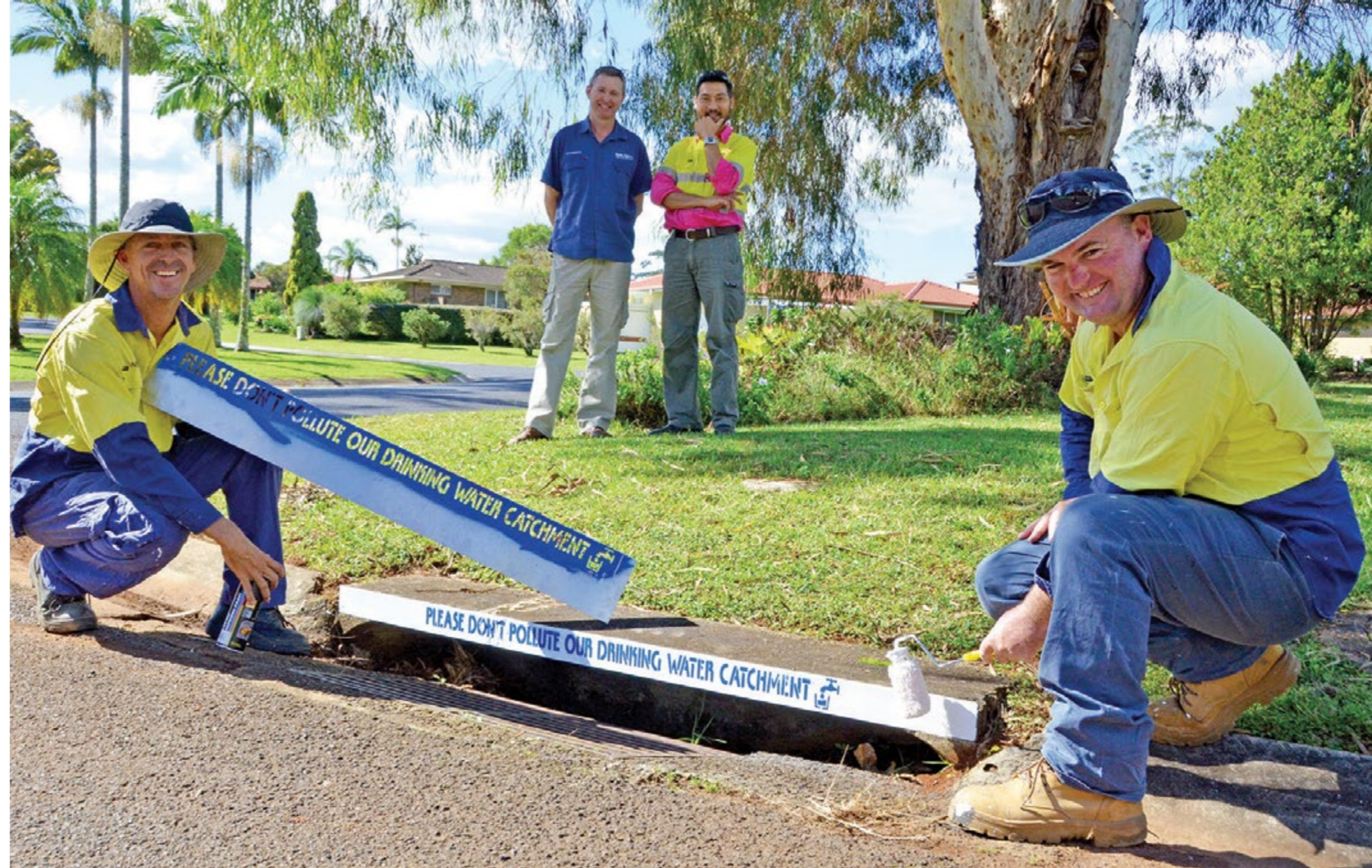
Lismore City Council Signs and Line Marking Leading Hand Neil Whiteman and Skilled Labourer Steve Murada (front) with Rous Water Catchment Assets Manager Anthony Acret and Lismore City Council Environmental Strategies Officer Anton Nguyen.
