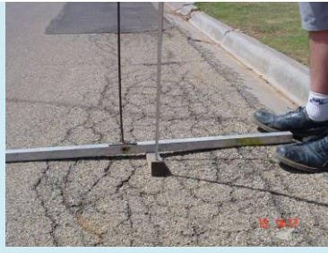
Typical pavement defects
