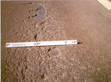
Typical surface defects
