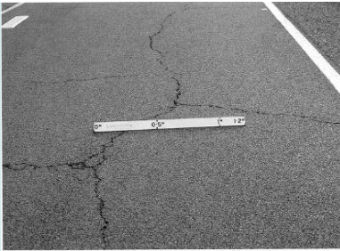
Typical road cracking
