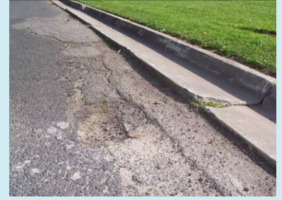
Typical local defects
