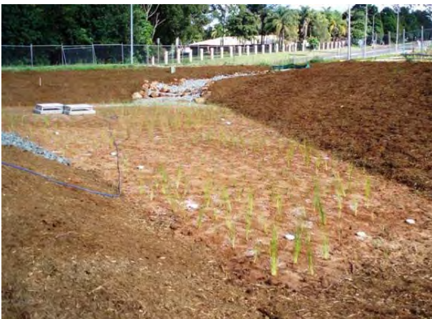
Bio-detention system beds at GSAC.
