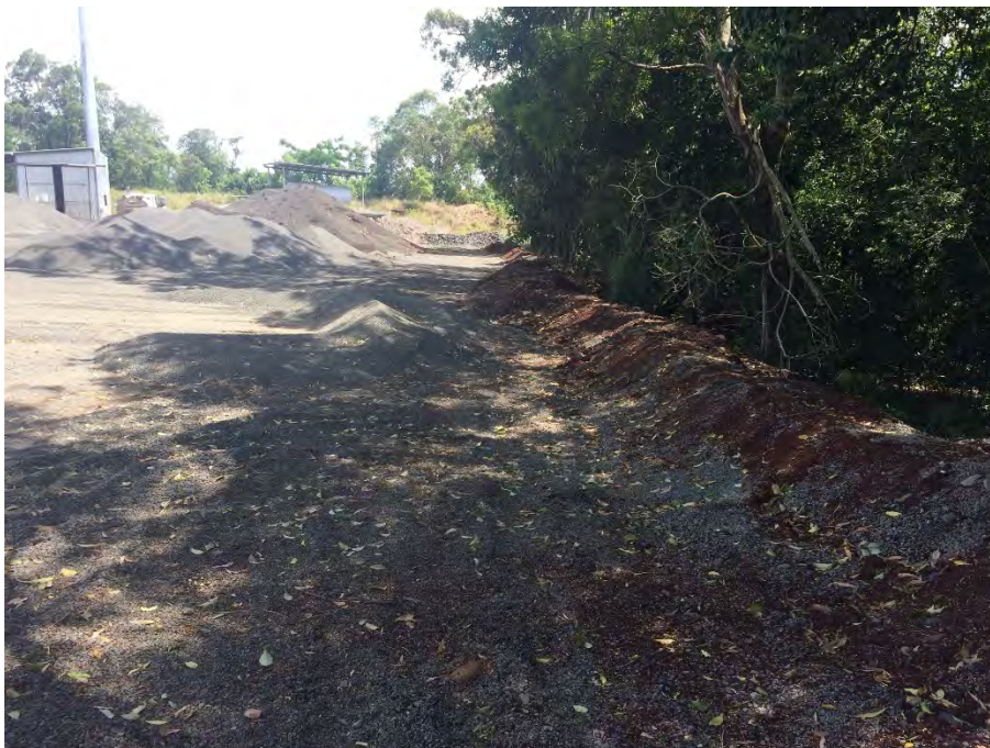
Plate 8: Dirty surface water containment bund
